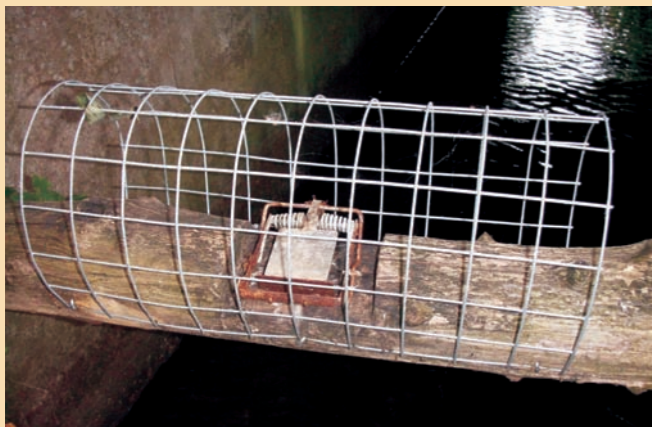
The wire mesh installed here is providing inadequate protection to non-target animals
