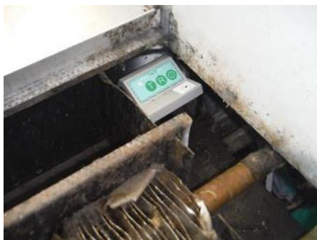
Detector mounted on a bracket and installed into a heating conduit
