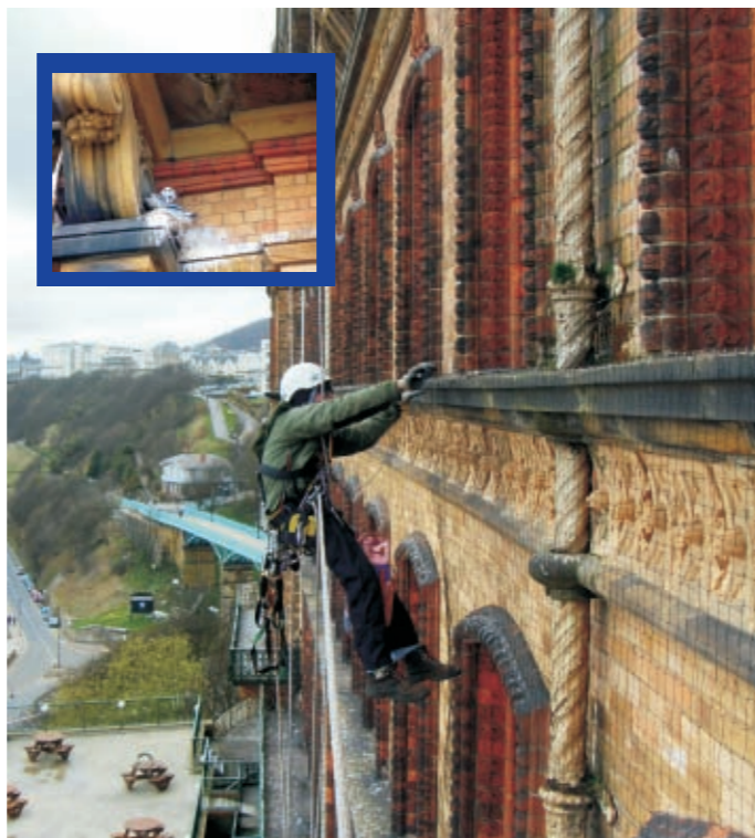
Abseiling proved the best way of installing bird netting on the façade of Scarborough's Grand Hotel. Inset: Before installation, nesting Kittiwakes caused damage and were a nuisance to guests
