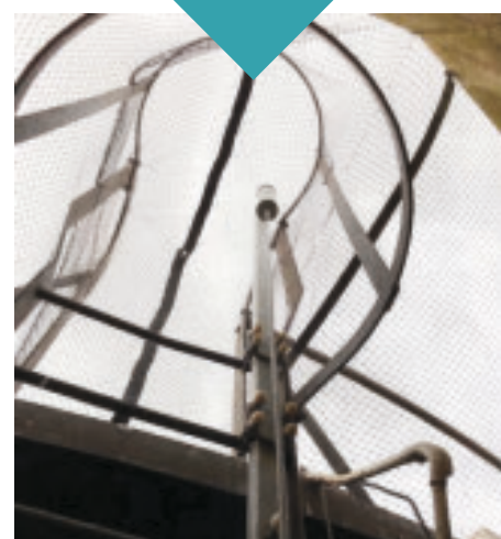
Zips were installed to give engineers access to the communications masts on the tower
